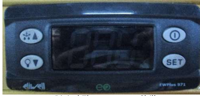
Digital Thermometer Chiller (Termometer Eliwell)
